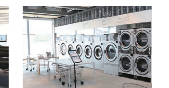
Laundry: A hygienic environment is maintained, such as by ensuring an emergency water supply and supplying emergency power for washing clothes.
